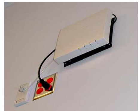
Wireless access point in one of the records storage bays at the new Plano ISD records warehouse
